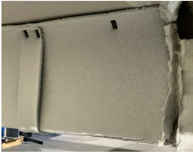
写真-12 出隅部のひび割れ Photo.12 Cracks on outside corners
