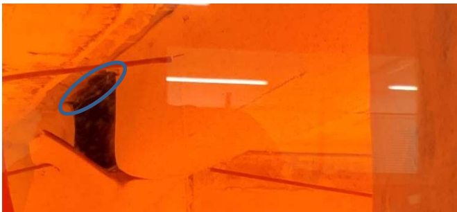
写真-6 被覆材が脱落した箇所 Photo.6 The part where the reflective coating fell off
