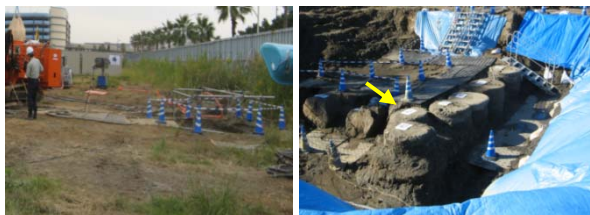
写真-1 実験現場状況（地盤改良前と改良後） Photo 1 States of the experimental field (before and after the ground improvement)
