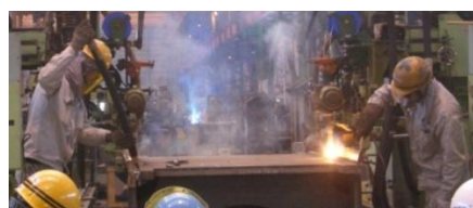
写真-8 実大溶接施工試験の状況例 Photo.8 Example of factory weld construction test
