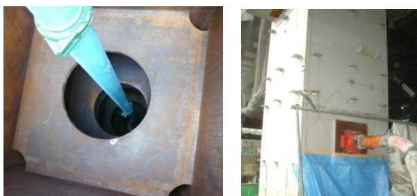
写真-6 落とし込み工法（左）と圧入工法（右）の状況 Photo.6 Dropped castion method (left) and pump up method (right)
