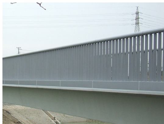
写真-2 ステンレス製の地覆カバーとアルミ鋳物高欄 Photo 2 Curb cover of stainless steel, and balustrade of Aluminum cast metal
