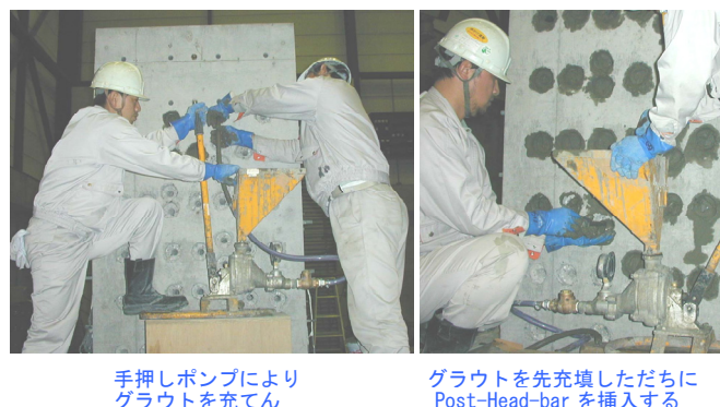
図-10 可塑性グラウト注入と Post-Head-bar 配置 Fig.10 Pre-grouting and inserting of Post-Head-bars
